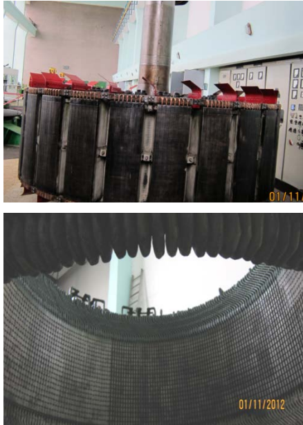
Fig.6. The hydro generator (rotor generator and fixed coil generator)
