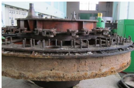
Fig.3. Turbine cap and the wicket gate control system
