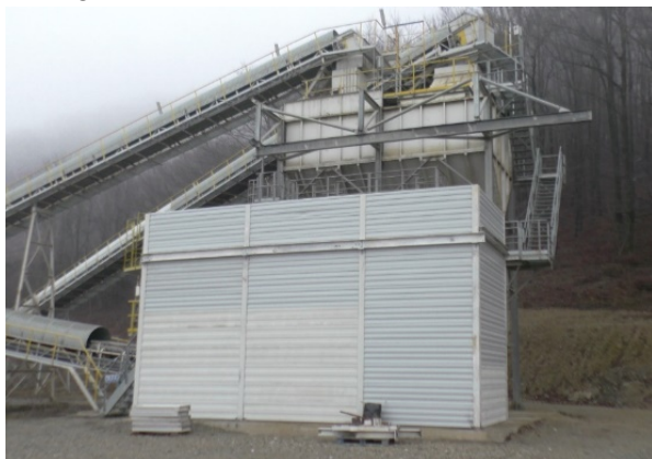
Figure 2. Noise barriers at crushers
