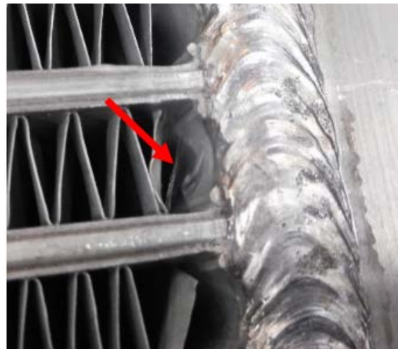
Figure 11. Damage of the cooler
