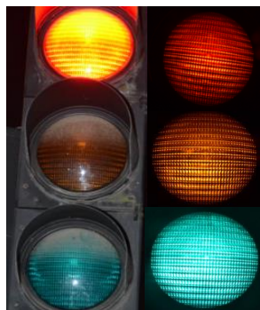
Figure 2. LED traffic lights before and after cleaning
